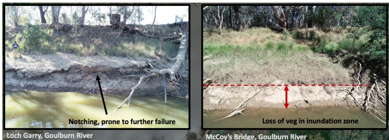
Figure 1. Bank erosion and loss of vegetation are related to flow operations, and verifying this relationship requires spatially explicit methods.
